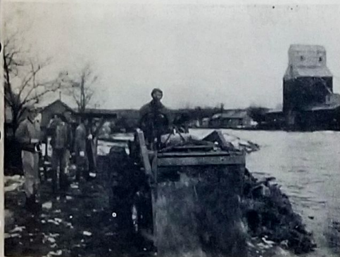
BOB HEIDEMAN, operating scoop tractor, dumps straw along edge of drainage ditch to protect NP dwellings on westside flat. The shovel brigade is at left.
